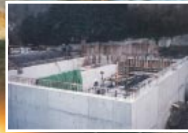
▲ The underground control structure in Crumplehorn Car Park
