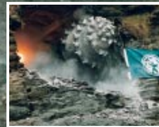
▲ 'The final tunnel breakout is a historic moment in Westcountry engineering' said Julian James, Environment Agency Project Engineer
